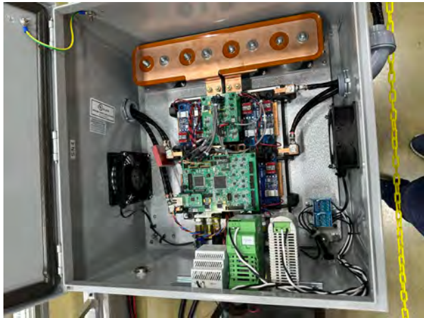
Assembled and tested 200 kW primary side HF inverter
